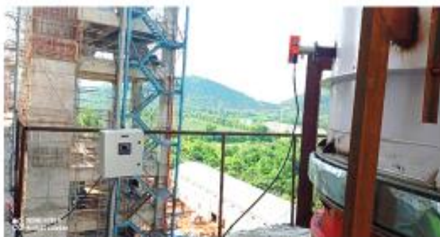
PM Analyzer at Cement Mill Stack
